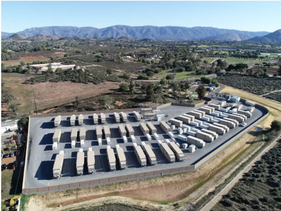
Terra-Gen’s Valley Center battery storage project opened in February 2022. A fire at the facility in September briefly shut down operations. (Terra-Gen)
